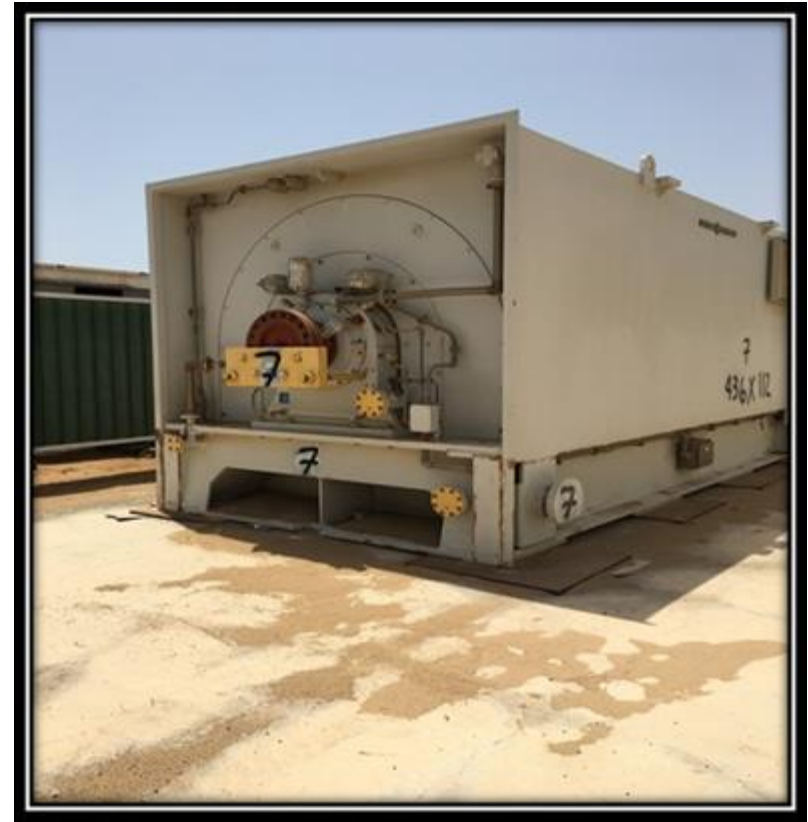
7EA Gas Turbine Generator
