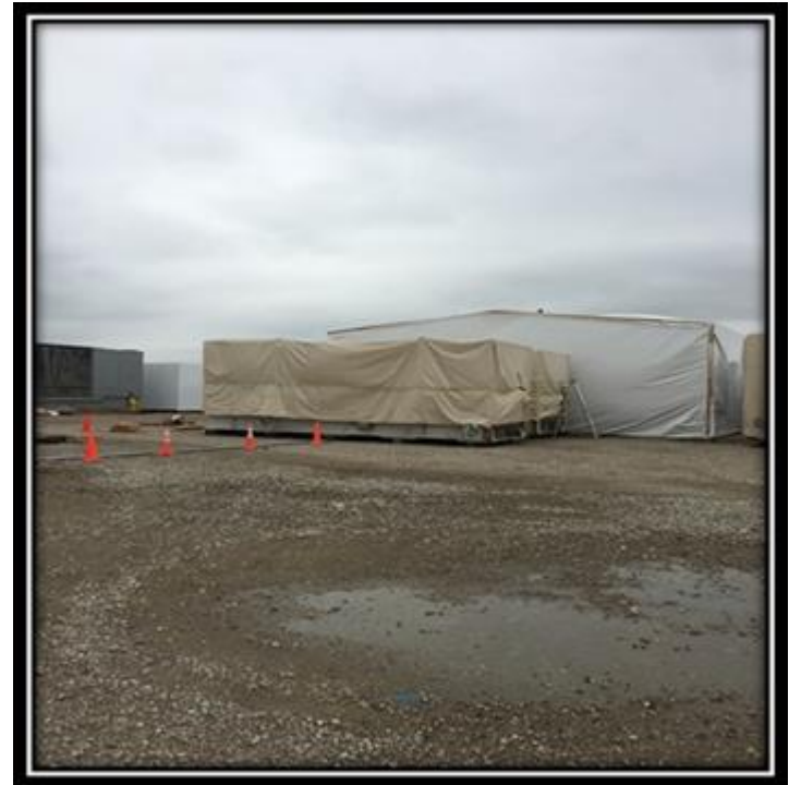
7EA Gas Turbine Generators Under Preservation
