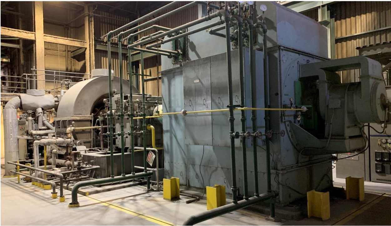
The turbine generator condenser is complete with all associated equipment
